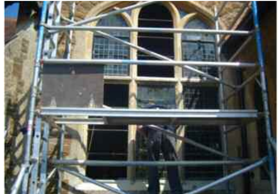
The windows being removed by a team from Sheppard Glass, hopefully they will be restored and refitted by the end of May.
